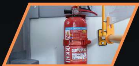
Fire Extinguisher Provision
